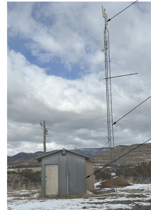
'A' EX. SHELTER & TOWER PHOTO
