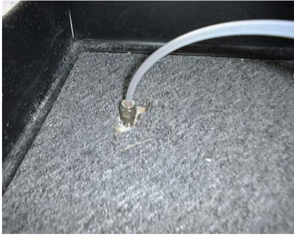
Figure 7. Compression fitting to probe
