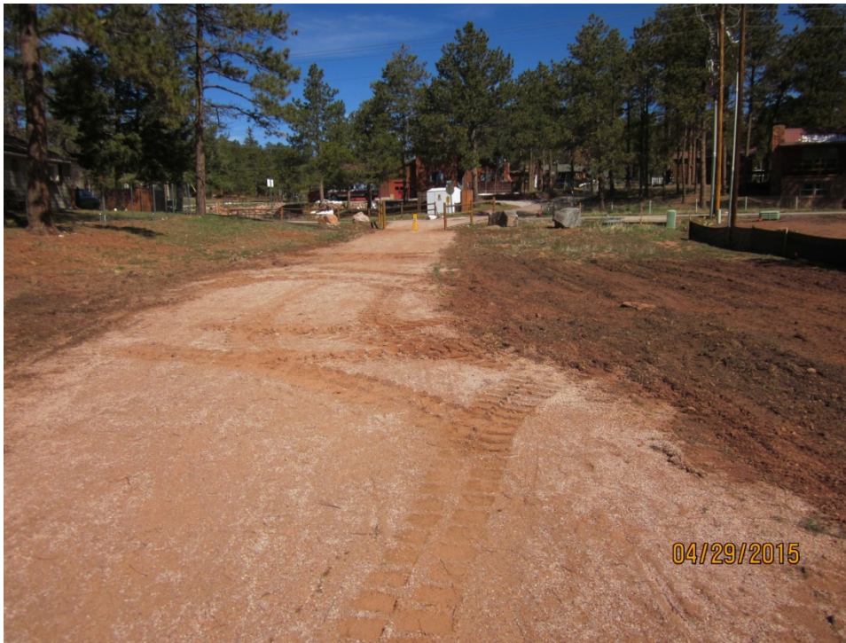
Before & After: Photos of the Fountain Creek Stabilization and Erosion Control project funded by a 2010 Pre-Disaster Mitigation (PDM) grant. The photos above are looking north, just south of Sheridan Avenue in Woodland Park.
